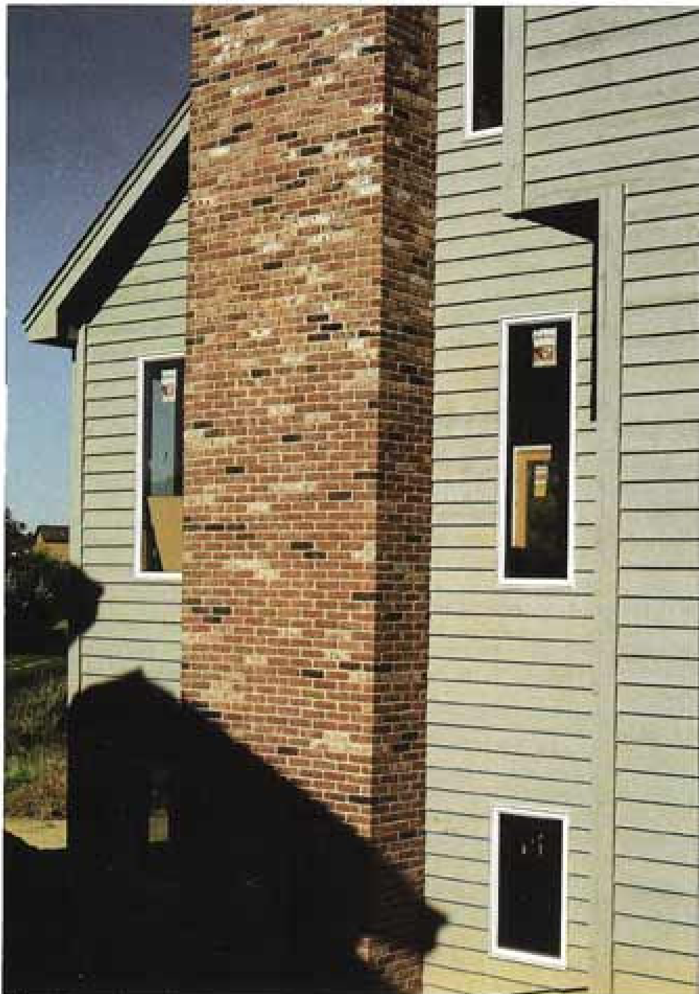
After 1 day of work, colors are blended to the satisfaction of the owner and builder. The color-treated brick are virtually indistinguishable from untreated brick and are guaranteed for 25 years.
